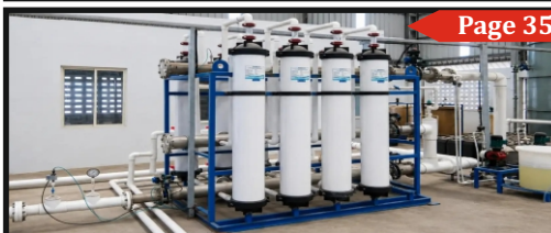
Water Filtration Plant
